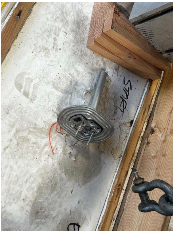
Photo No. 9 Typical Joist Condition Failure of OmniShield™ Assembly
